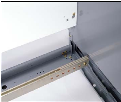
Figure 26: Ground Bar Bolt Removed
