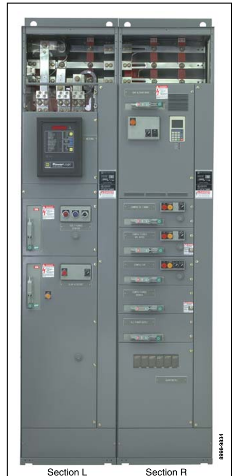
Figure 6: Two-piece Bus Barriers Removed (splice connection made)
