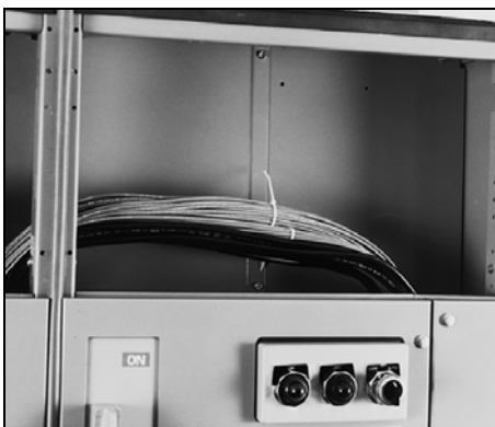
Figure 29: Wiring in the Top Horizontal Wire Trough
