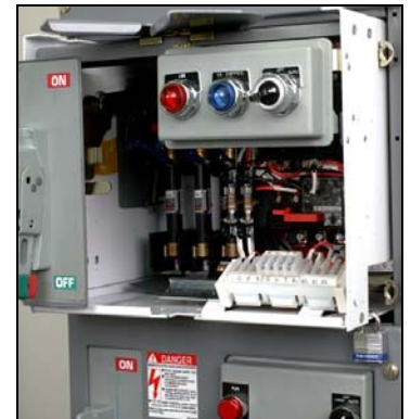
8998-9639 Figure 45: Locked Out Device
