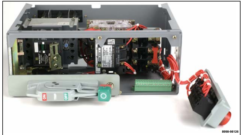
Figure 51: Control Station Plate Removed
