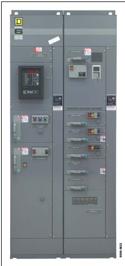
Figure 4: Motor Control Center
