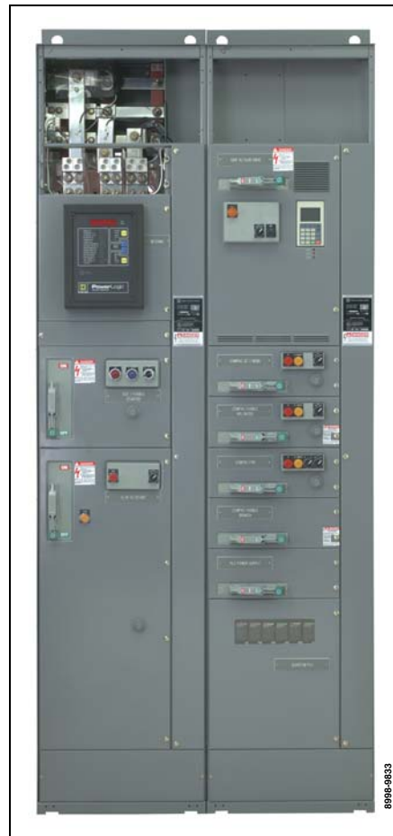
Figure 5: Top Horizontal Wire Trough Covers and Main Lug Unit Door Removed
